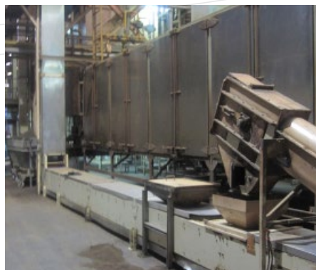
Ewos – Chile Simatek Universal Elevator in connection with pellet drying
