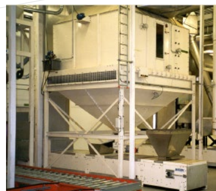
Polar Feed – Norway Simatek Universal Elevator in connection with pellet cooling
